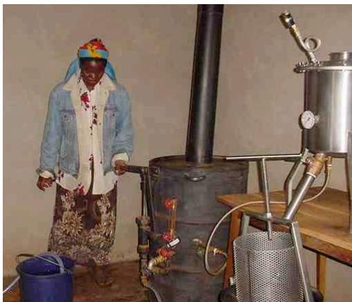
Filling the boiler from a bucket, Mozambique ←
